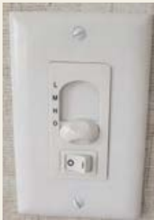
Wire & Brace W/ Switch Only For Ceiling Fan
