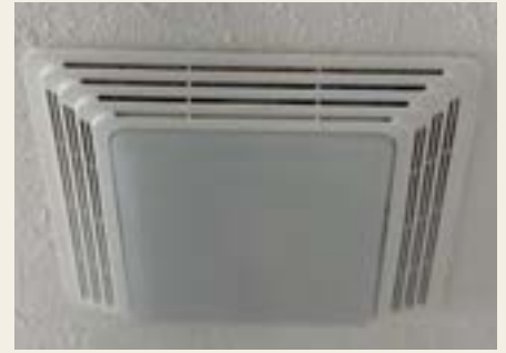
Exhaust Fan W/ Light
