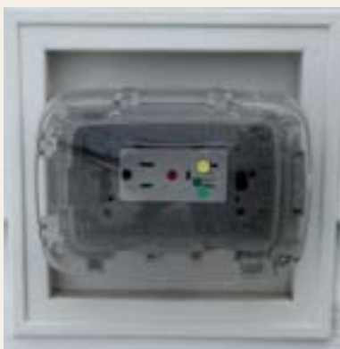
Exterior GFCI Receptacle
